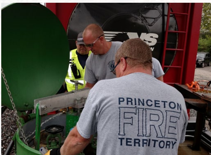
Cris Burch (Norfolk Southern) watches as firefighters from Princeton Fire Territory place a Chlorine Institute Emergency C kit.
