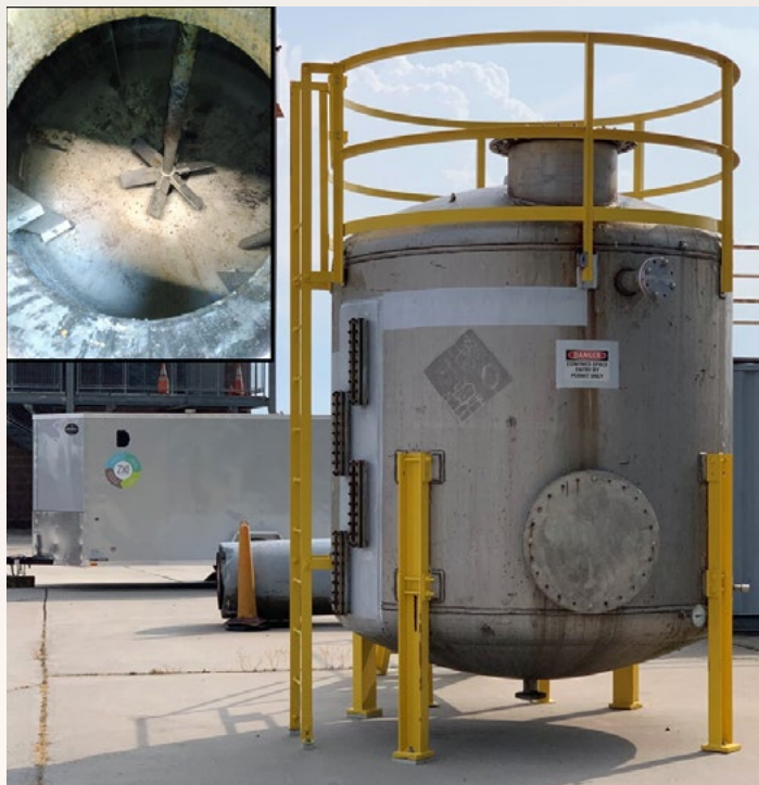
Figure 4: A chemical reactor can pose several technical challenges with heights, limited access, mechanical agitators (see insert), as well as the chemicals used in the reactor.
